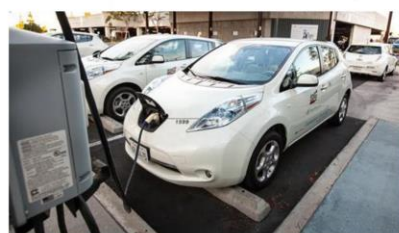
EV station (source: San Diego Gas & Electric)
