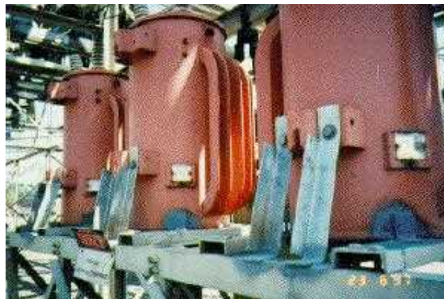
Figure 5-11: Direct bracing of equipments' body for controlling overturn and slippage damage modes
