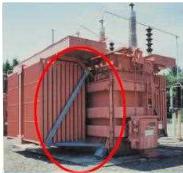
Figure 5-5: Reinforcing bracing of transformer's radiator
