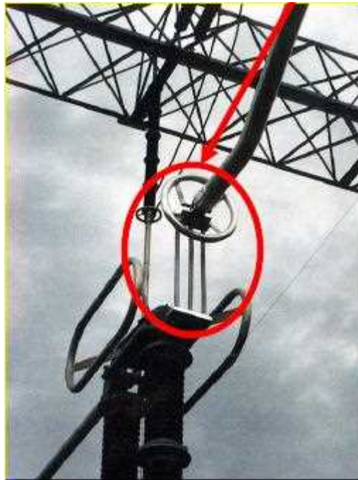
Figure 5-8: Embedding cut-off switch for controlling equipment's performance
